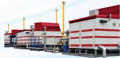
Gas-Set Compressor Stations
