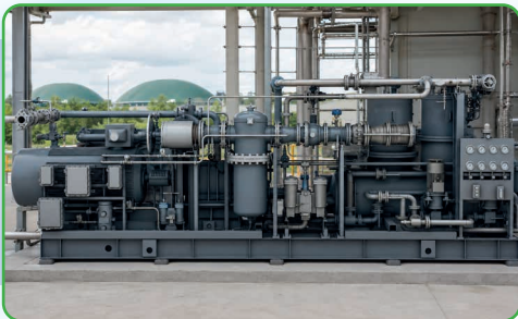
Biogas Upgrading Compressors
